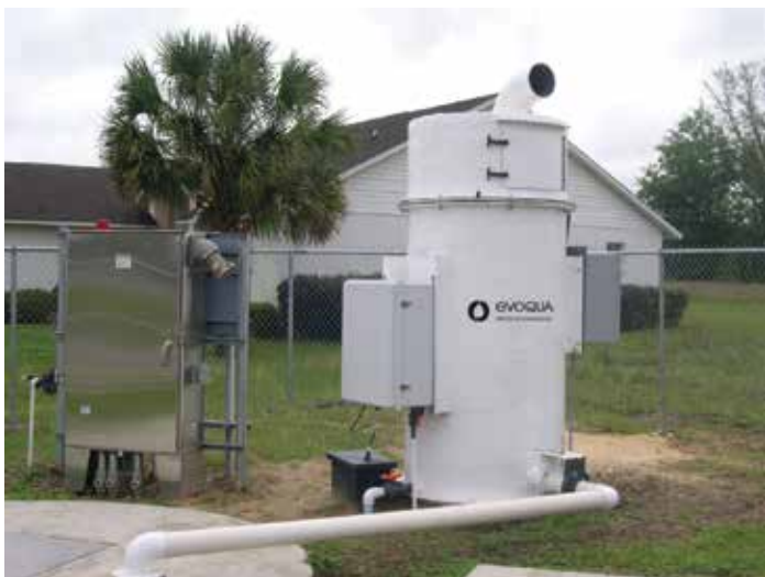
With a manufactured biological odor control system, media instability is reduced and control issues are limited. (ZABOCS® Biological Odor Control System)
