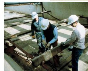
Installation and aftermarket services are available to plant operators and managers to help protect equipment and the investment in utility assets.
