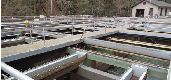
Chain and scraper system components, drive systems, and scum pipes replaced in the Grass Valley, California wastewater treatment plant.
