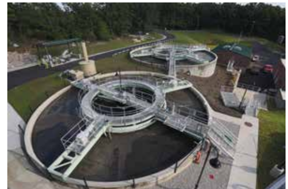
BioMag® system increased plant capacity from 0.75 to 1.6 MGD without adding additional bioreactor or clarifier tanks.
