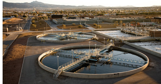
Circular and Rectangular Clarifiers
